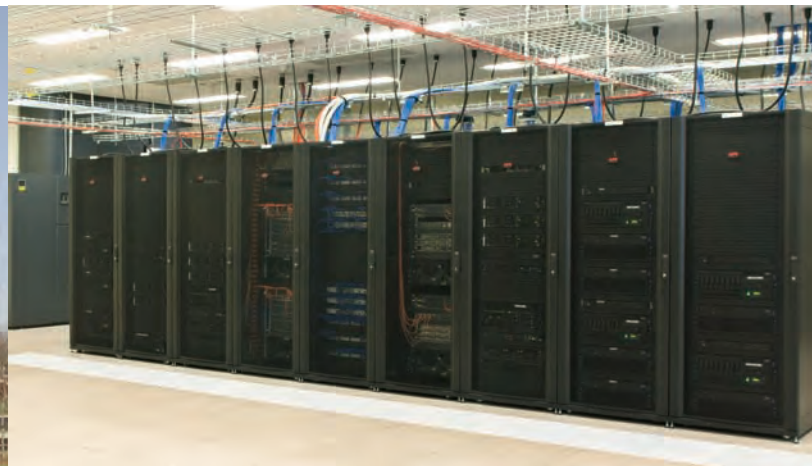
Data Center: Montana State Fund, Helena, MN, 2,000 ft 2
