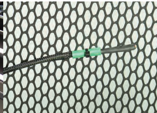
Sensor Mounted to the Face of the Rack for SmartAire & PowerAire
