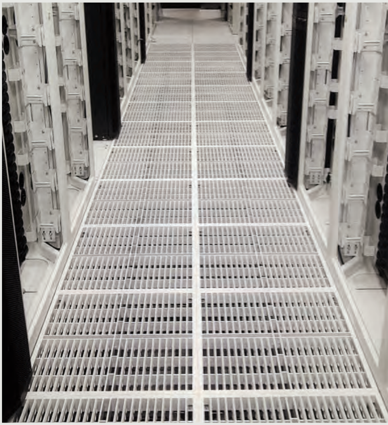
Data Center AT&T, New York, NY, 25,000 ft 2
